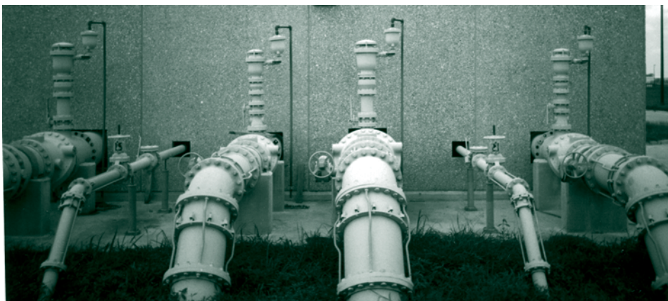
Surge-Suppression Air Valves and Isolation Valves in a pump discharge application.
